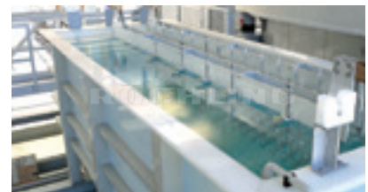
Polystone® P homopolymer natural Anodisation basin for treating door handles
