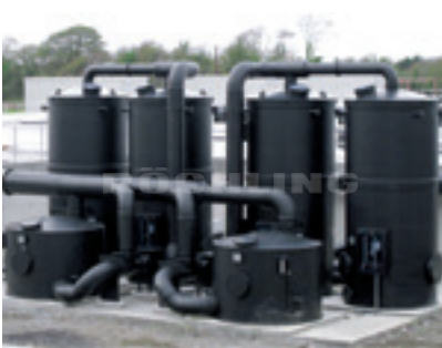
Polystone® G black B 100 Air purification system in a water treatment plant
