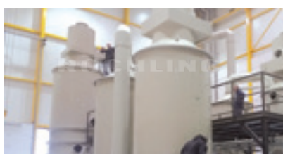
Gas scrubbers in a biogas plant made from Polystone® P homopolymer grey
