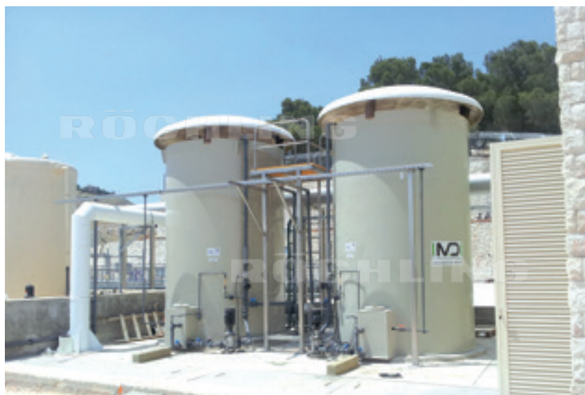
Bio filters for odor neutralisation
